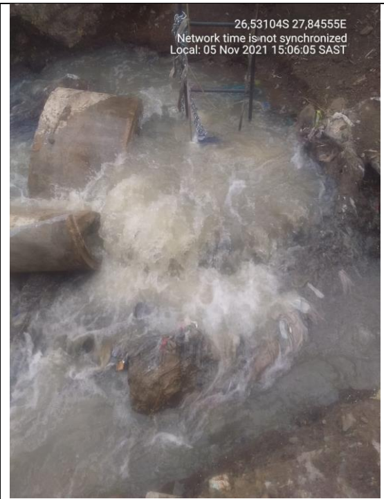
Figure 4: "Popped" Manhole Upstream of Rescue Site due to Overpressured Line
